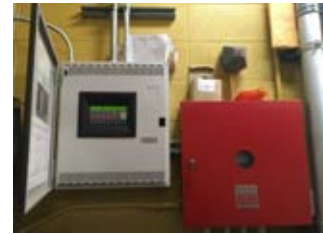
Fire Alarm Control Panel
