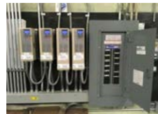
New Panelboard and VFD's
