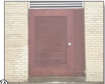
⑦A HOLLOW METAL DOOR & HOLLOW METAL FRAME; STAFF INDICATED SCHEDULED FOR REPLACEMENT
