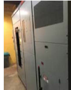
Main Electric Service
