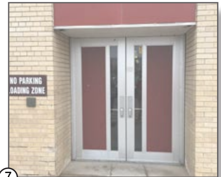
⑦ ALUMINUM DOORS & ALUMINUM FRAME, STAFF INDICATED SCHEDULED FOR REPLACEMENT
