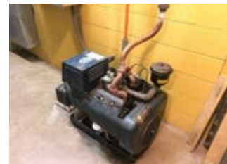
Existing Emergency Generator
